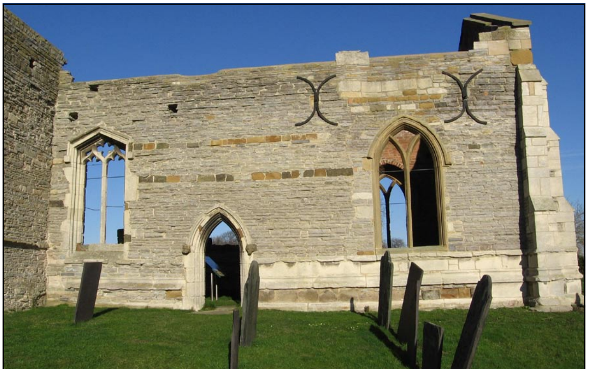
Figure 16. The south wall of Chancel with its repeated repairs.
